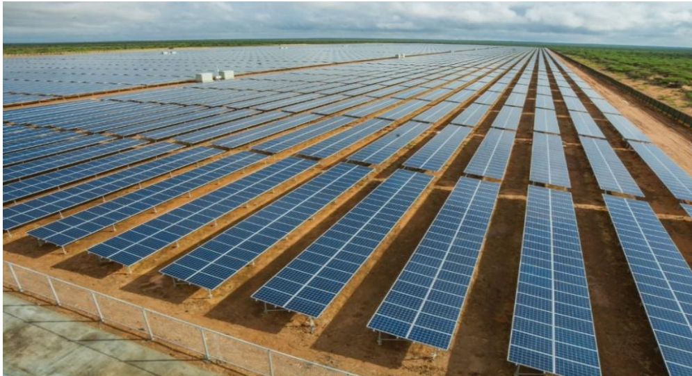
An aerial view of the Solar panels at the plant
