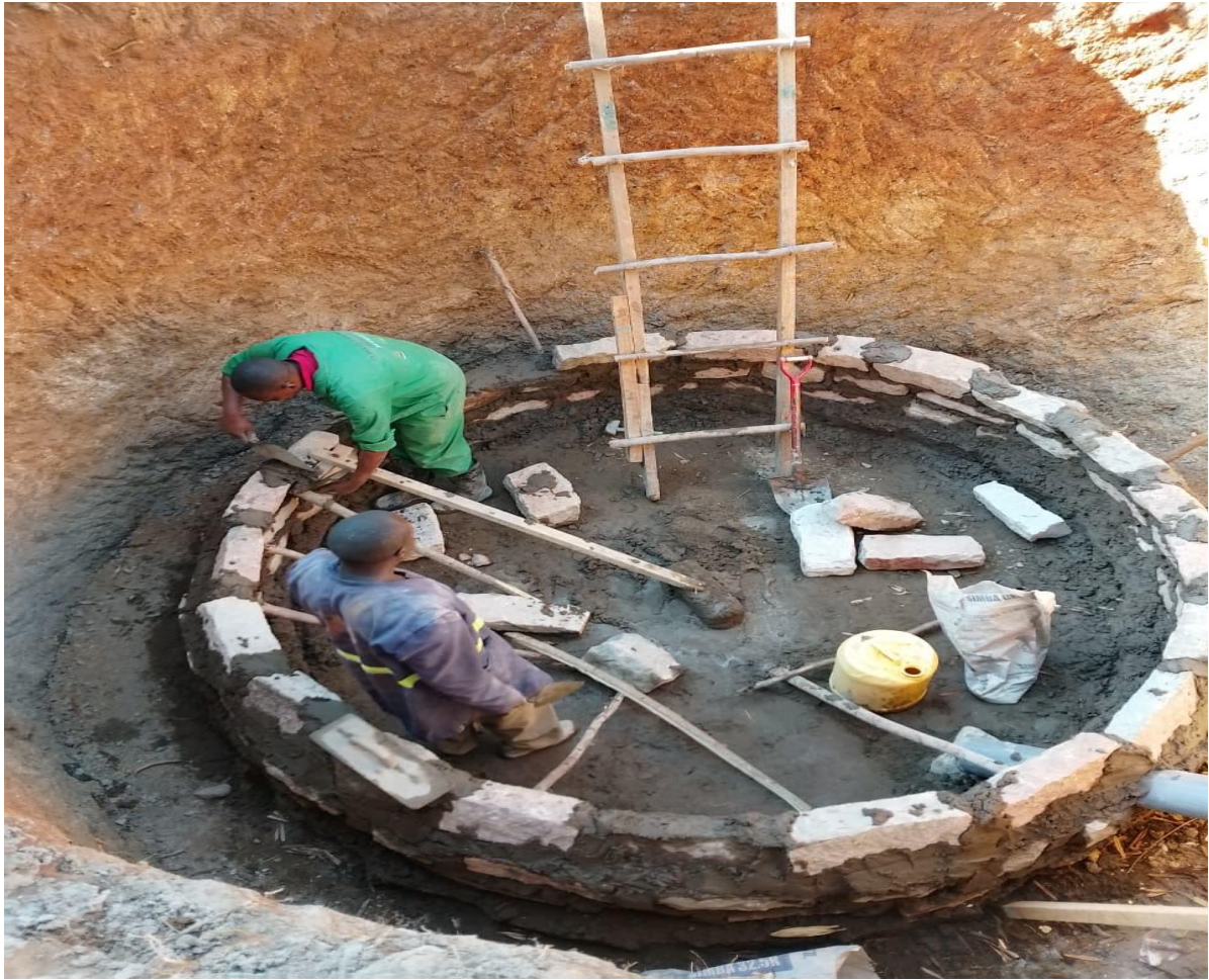
Fig 6: Biogas installation by Energy Centres artisans
